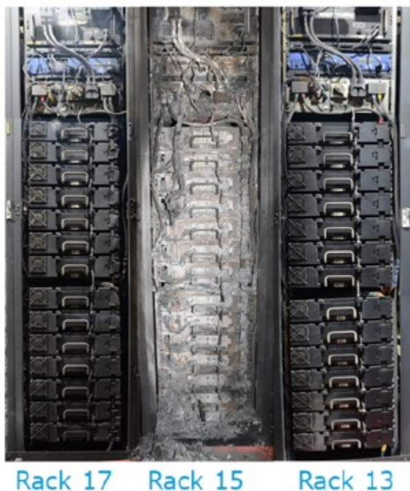
Figure 13: Destruction of Rack at McMicken.
