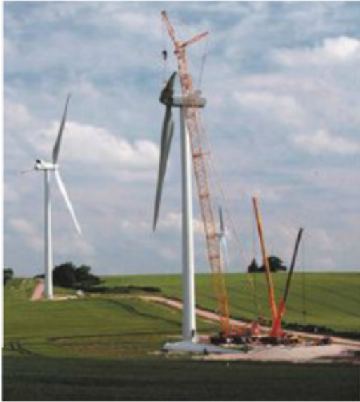
Turbines being constructed by RES at a wind farm at Wadlow, Cambridgeshire, about three years ago.
