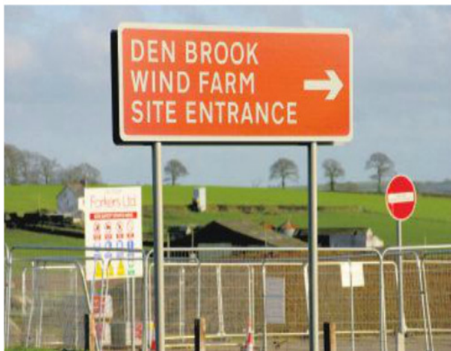
The entrance to the Den Brook wind farm site off the A3072 between Bow and North Tawton. AQ 8767
